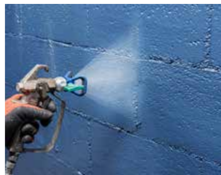
... unplastered walls, and
